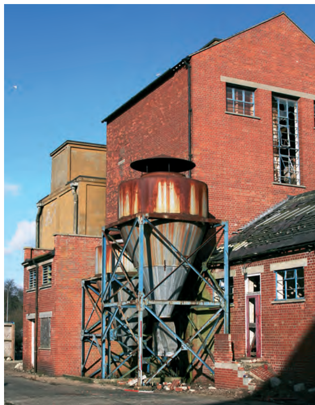
Plate 3 Ditchingham Maltings: the western elevation of the loading bay and plant room.
